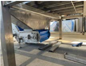
Conveyor belt for ice extraction
