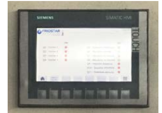
Siemens touch panel for the control and adjustment of all operating parameters
